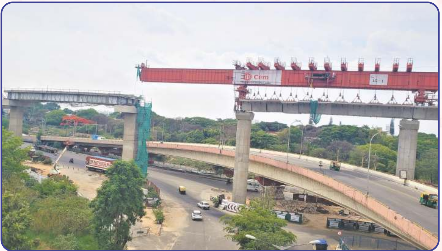
Metro Pier ID BP90-BP91 (Near Outer Ring Road Flyover, K. R. Puram)
