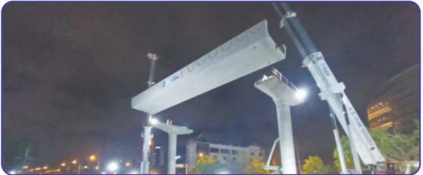
1 st U-Girder launched at Doddanakundi on 18.06.2022 of Phase-2A (Package 2) of ORR Line.
