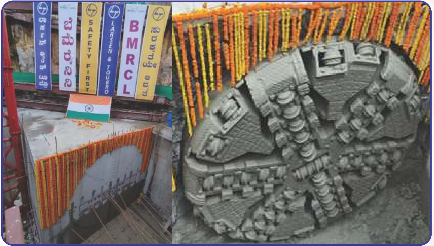
TBM Vindhya, between Cantonment and Shivajinagar Metro Station made a breakthrough at Shivajinagar Metro station on 13.10.2021.
