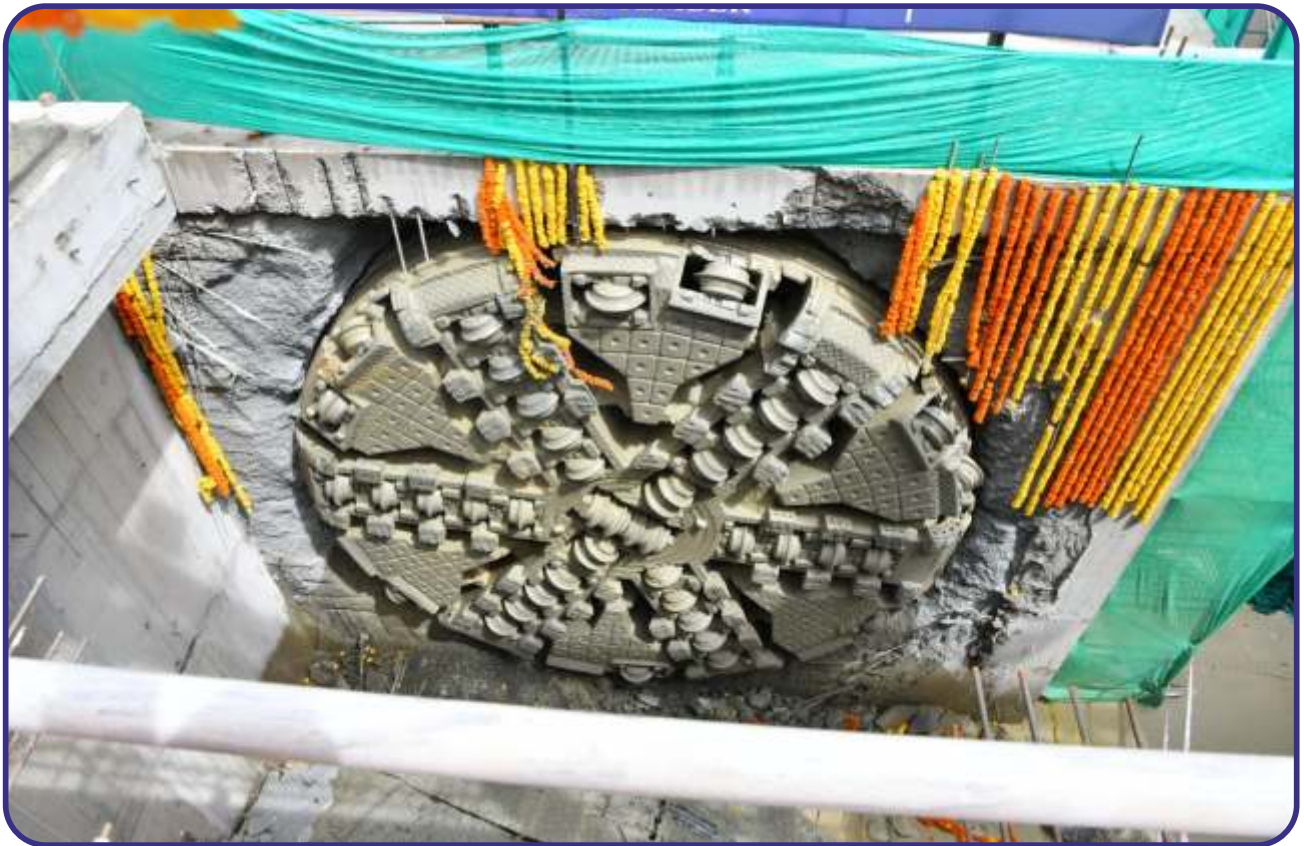
1 st TBM Breakthrough (URJA) between Cantonment Metro Station and Shivajinagar Metro Station was at Shivajinagar Metro Station on 22 nd September 2021. Shri Basavaraj Bommai, Hon'ble Chief Minister, Government of Karnataka along with other Hon'ble Ministers witnessed the breakthrough.
